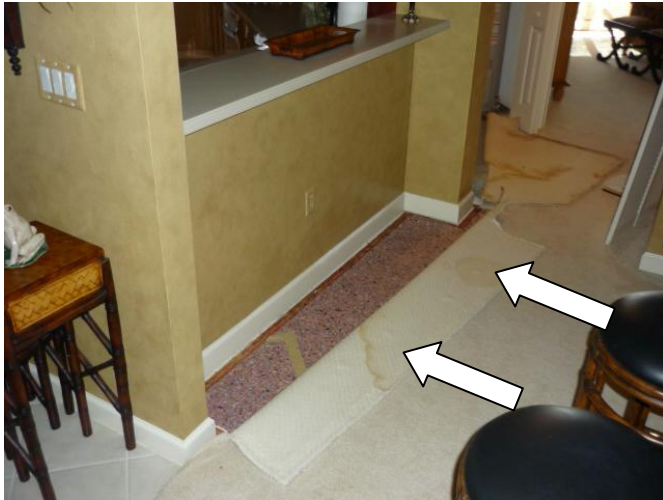
Moisture stained carpet where the kitchen bar stools are located
