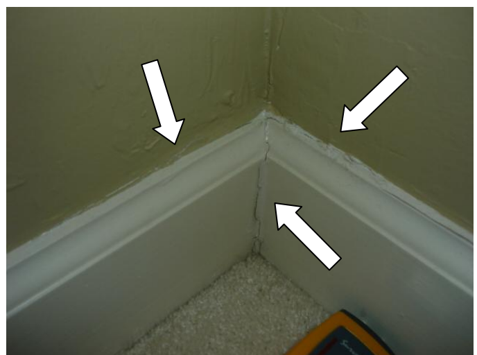
Photos shows minor water damage at the baseboards in the guest bedroom closet
