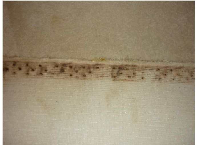
Moisture staining/rust on the carpet backing
