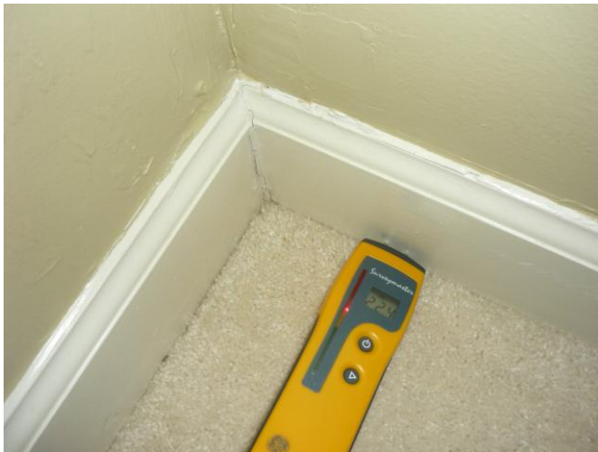
Elevated moisture content from the area shown above
