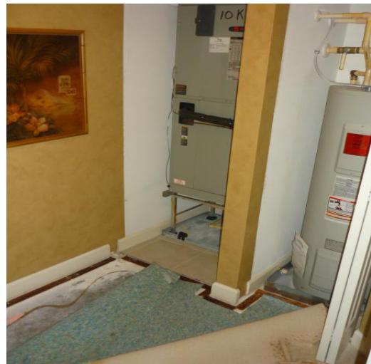
Area view of the air-handler closet
