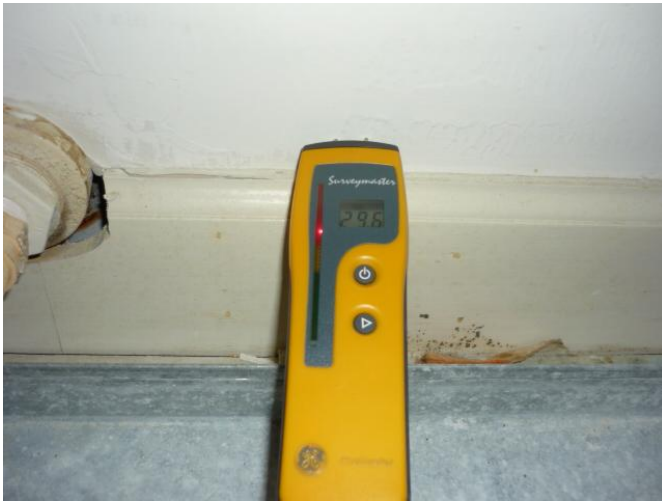
Water damage and elevated moisture content from the air-handler closet
