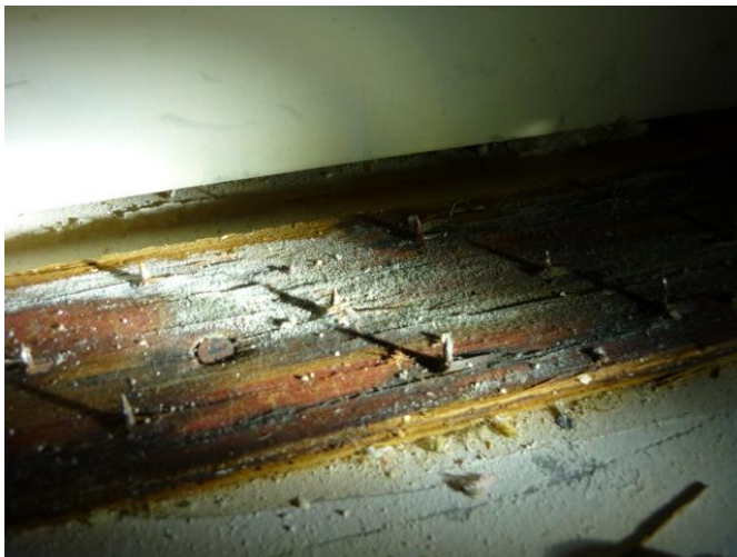
Water damage and suspected mold growth on the carpet tack strips
