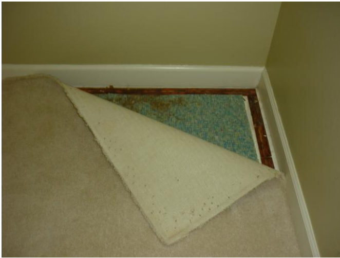
Moisture staining on the carpet backing and pad in the guest bedroom closet
